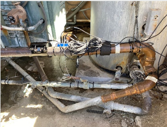
Electronic monitoring of water heater load. Photo credit: AEA
