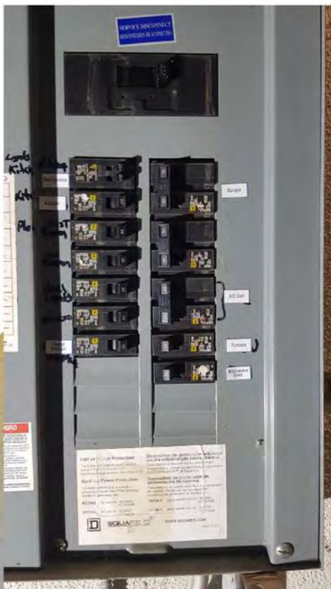
Note unused slots
