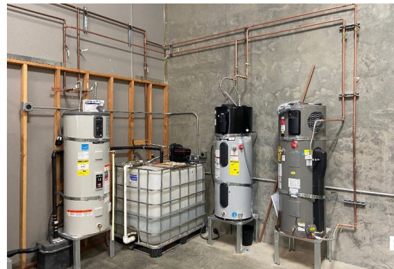
Figure 15: Heat Pump Water Heater Training Center – DeHart Technical School
